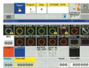
Check of interface panel
